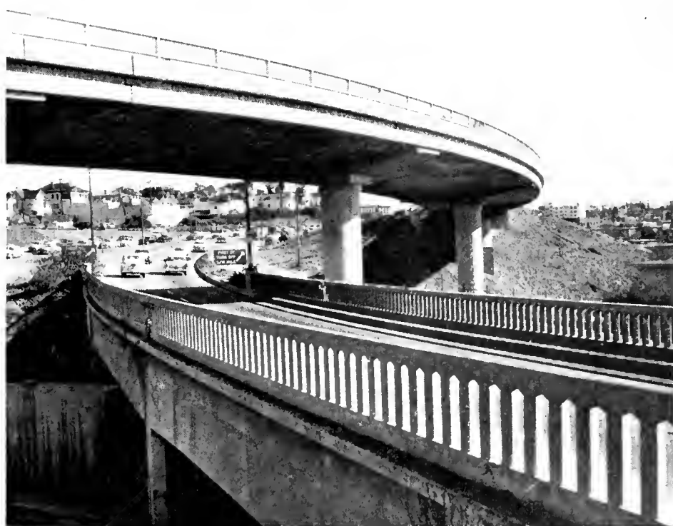
Prestressed span over the eastbound Santa Ana Freeway bridge and the on-ramp for the eastbound San Bernardino Freeway below, showing the three-level separation at this point. View also shows bottom flanges of the prestressed girders and the general shape of the girder step bearings.
